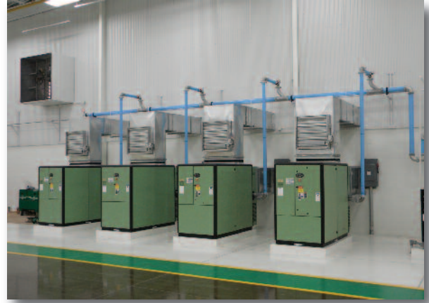
Transform your compressor room into a show piece
